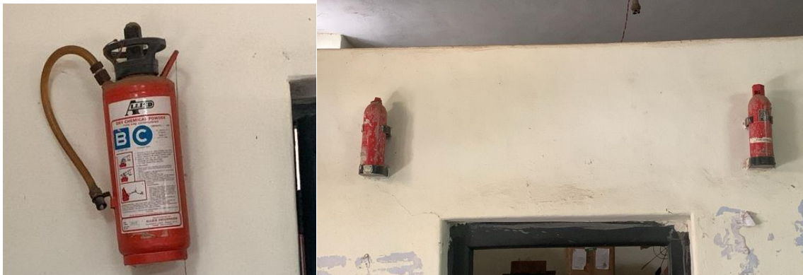
Fire extinguishers installed at college building
