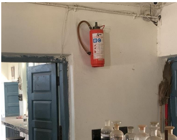
Fire extinguishers installed at college building
